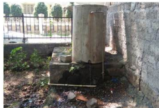
Water storage tanks are not well maintained
